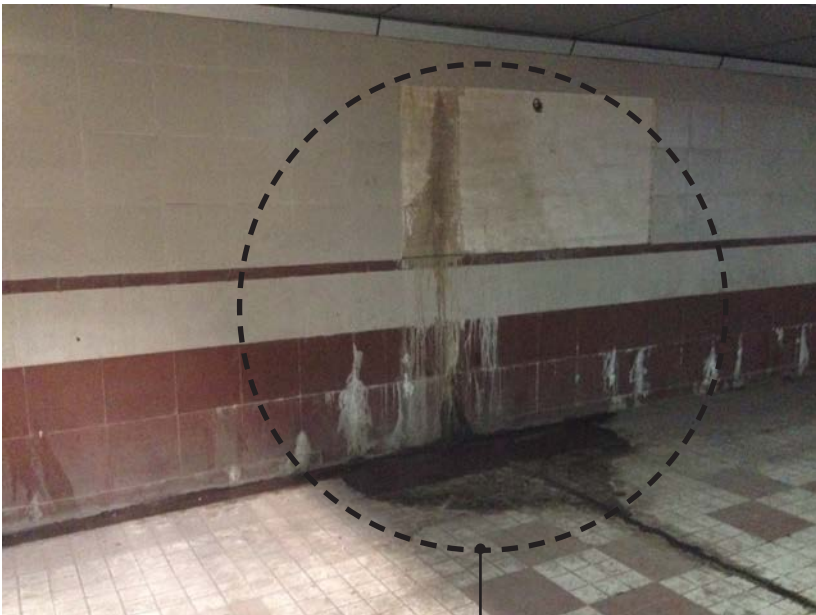
Subways are not very well maintained which further makes them unusable.
