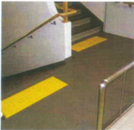
Photo 12 Continuity of Handrails
